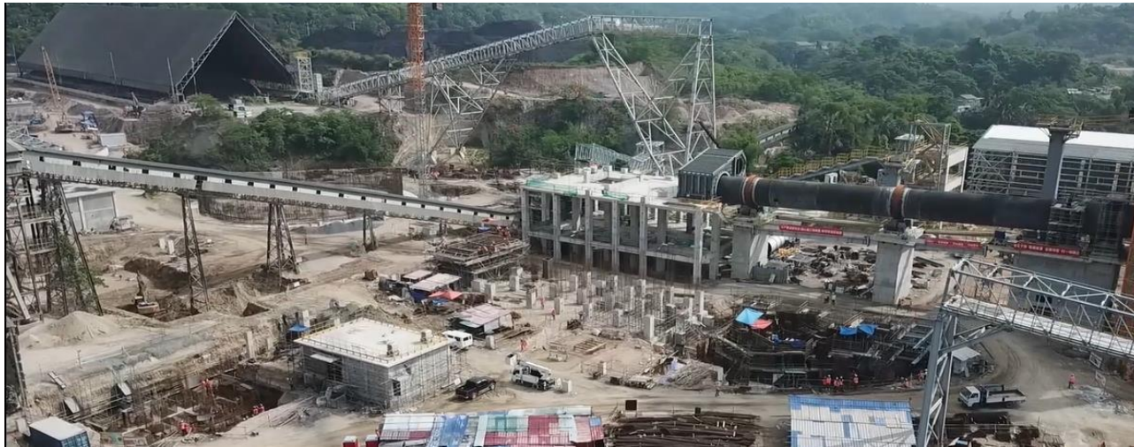
CBMI – NEW CEMENT PLANT 3.500 TPD – PHILIPPINES (VERY HIGH WIND AND SEISMIC CONDITIONS)
